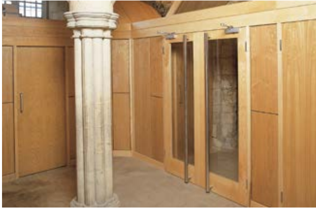
St Hilda's, Hartlepool Internal doors, a WC and boiler housing built within the west tower.
