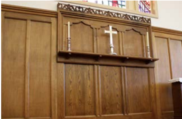
All Saints & Salutation, Darlington New panelling alongside converted panelling from the original church.
